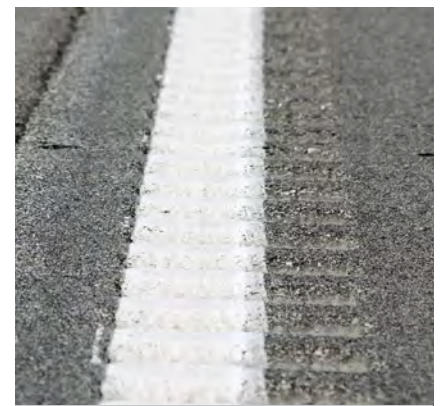
Example of an edge line rumble stripe.
